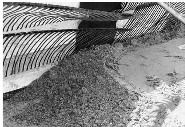
IMAGE T: Compacted select fill brought up to the level of the geogrid.
