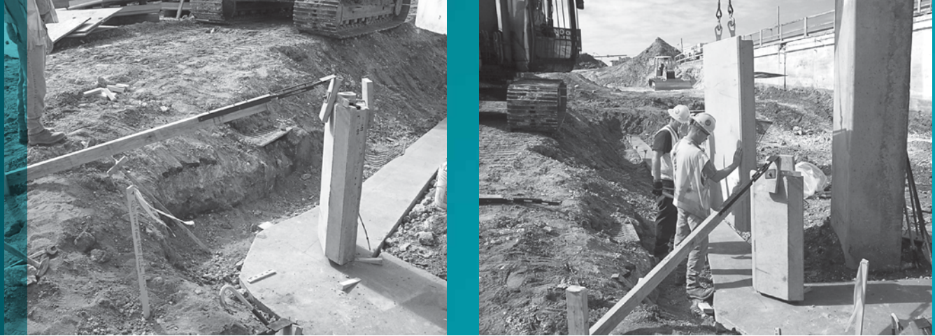
IMAGE E: Panel placement commonly begins at corner locations. Placement and bracing of concrete panels.
