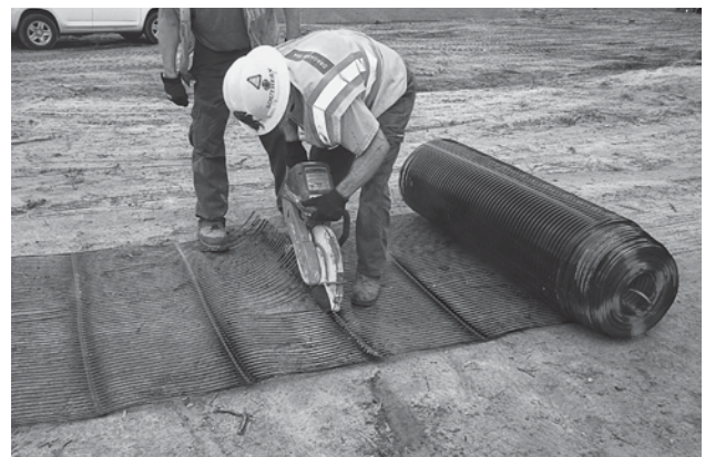
IMAGE D: Safe cutting of geogrid may be accomplished with a variety of cutting tools. Care should be taken to avoid cutting the transverse bar.
