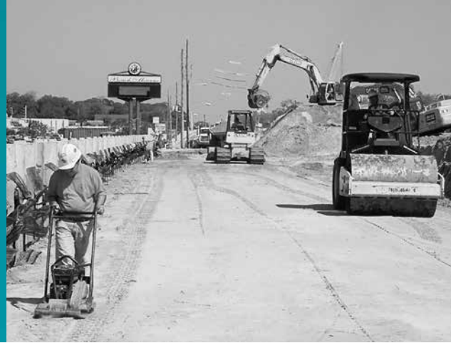
IMAGE R: Use only lightweight equipment to compact fill within 3 ft of ARES® panel.
